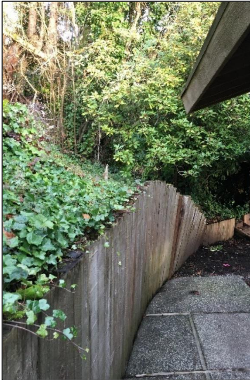
Photograph 1. Looking northeast at the existing yielding wall northwest of the existing residence.
